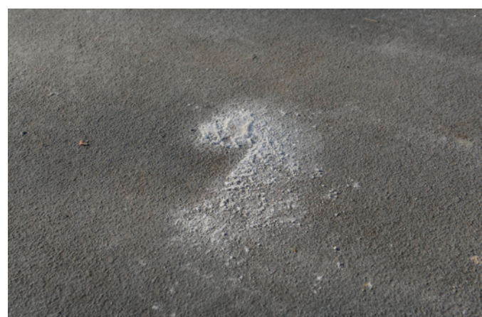
Particularly exposed to de-icing salt attack
