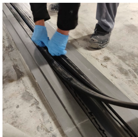
Gluing the rubber expansion element into the joint profile MC-Floor Connect CPS
